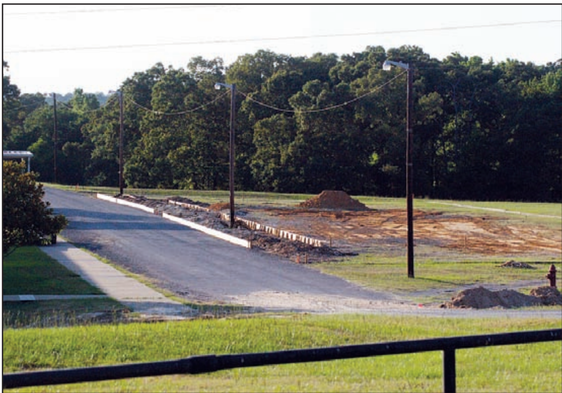
Forms are set to begin pouring a new parking lot at the junior high building, an improvement that came out of the Board's recent goal-setting meeting. Van 'Go' photo
