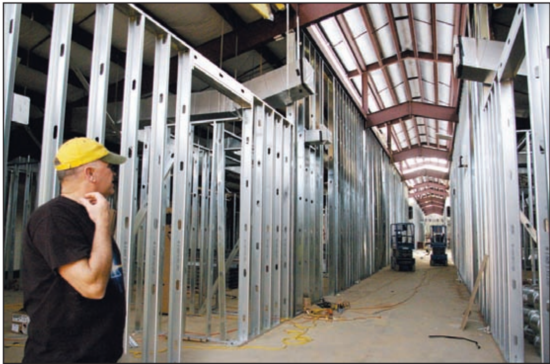
School board trustee Ron Goodwyn inspects an interior hallway in the first wing of classrooms. Van 'Go' photo
